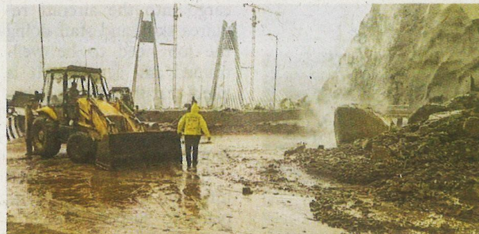
RESTORING A KEY LINK. Work on to clear the debris on the Pune-Mumbai carriageway of the Khopoli-Kusgaon 'Missing Link' following a landslide due to heavy rain PTI
